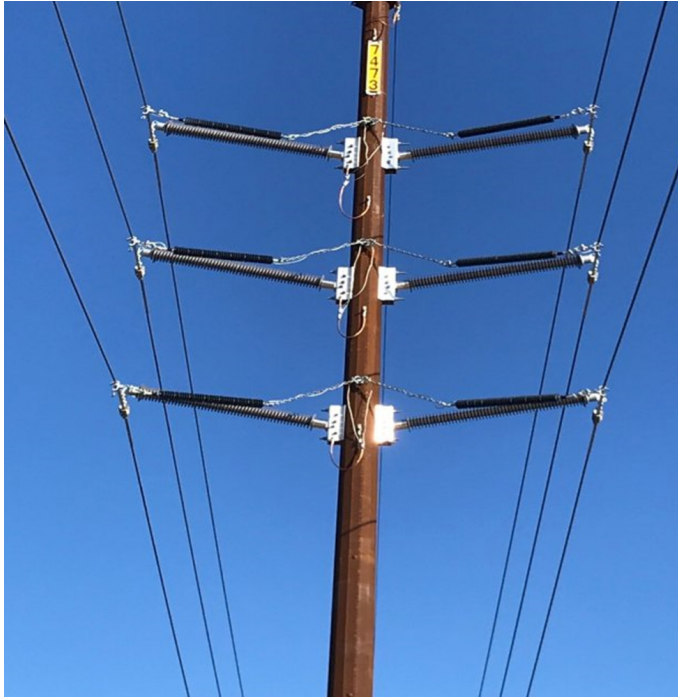
Figure 10: Innovative modeling method results in optimal placement of surge arresters; courtesy of PPL Electric Utilities.
