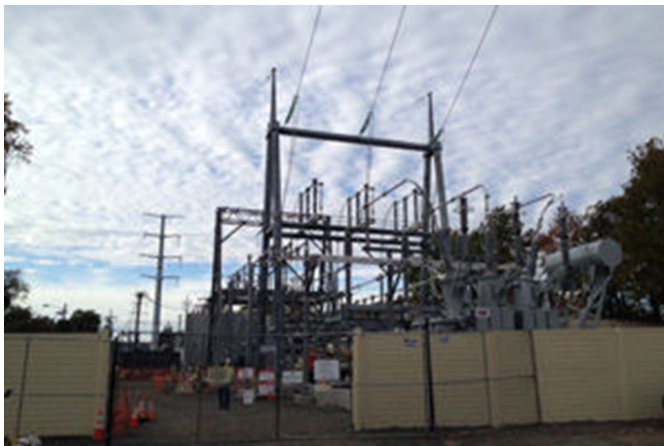
Figure 15: Fanwood Substation; courtesy of PSE&G.
