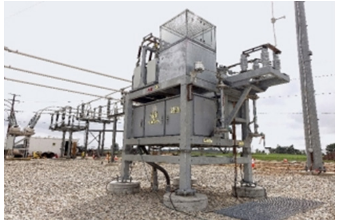
Figure 12: GIC blocker; courtesy of ATC.
