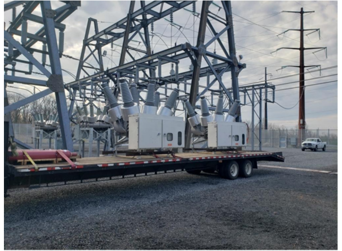
Figure 9: Delivery of the first 69kV vacuum circuit breakers to be piloted on PPL's system; courtesy of PPL Electric Utilities.
