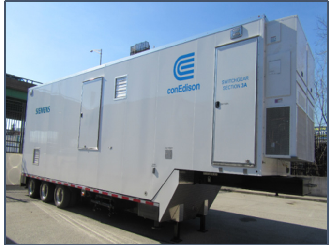
Figure 14: Mobile switchgear; courtesy of Consolidated Edison, Inc.
