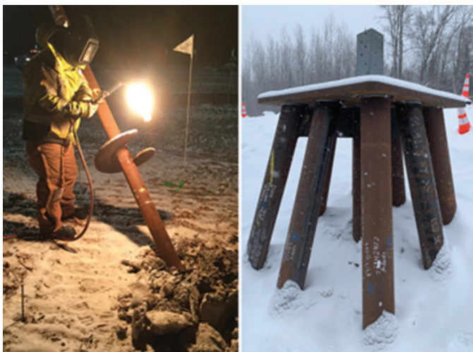
Figure 7: A crew member cuts a helical pile with a torch during night construction (left). High-reveal helical pile pedestal set on the side of a slope. The helical piles are welded to the pile cap which serves as the base for the transmission tower (right); courtesy of POWER Engineers Inc.
