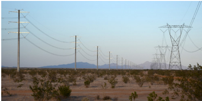
Figure 4: High-Voltage Monopole and Lattice Transmission Towers, California; courtesy of Argonne National Laboratory.
