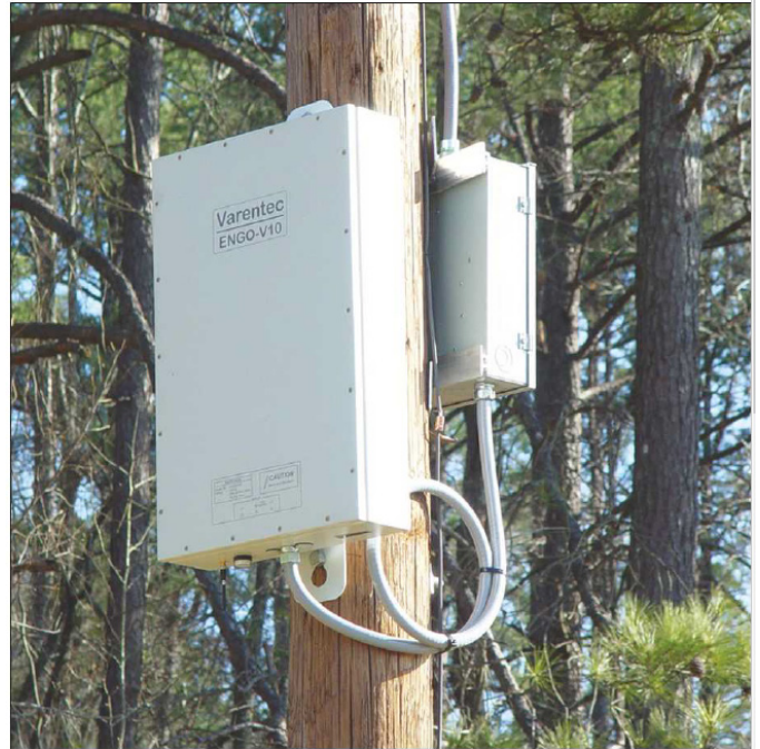
Figure 11: Installed ENGO unit; courtesy of Southern Company.
